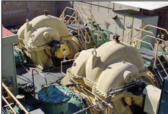
Cooling water pumps have been sealed leak free for over 9 years - Shaft size 300 mm (11.75 in.)
